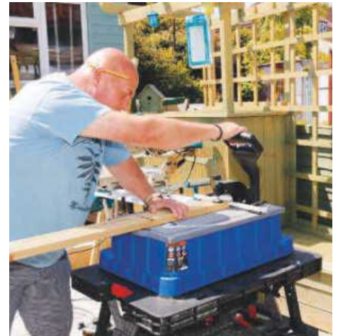
STEP 10. The long boards are drilled for pockets in the same way
